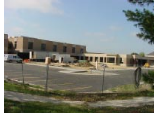
Law College renovation and additions will include a multifunctional courtyard on the north side and new building approach on the south. Planting will begin next spring.
