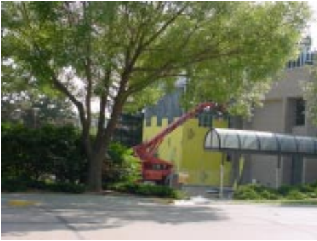
A small addition is under construction on the NE corner of the Barkley Center.
